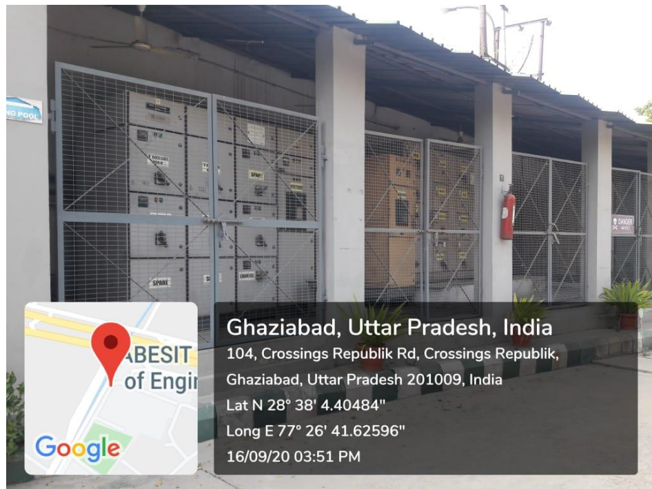
Figure-3.3: MCB Panel Room
