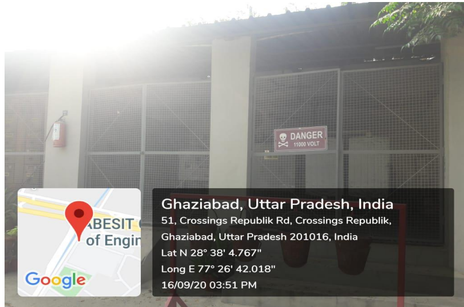
Figure 3.4: MCB Panel Room
